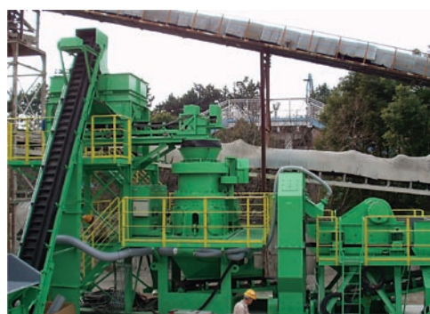
図6 設備全景 Fig.6 Whole view of equipments
